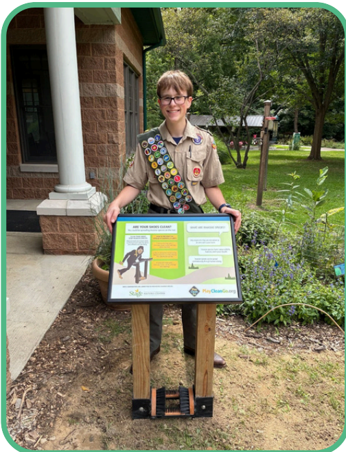
Alex Doerr poses with the PlayCleanGo Boot Brush Station he helped install as part of his Eagle Scout Project, Stage Nature Center, Michigan.
